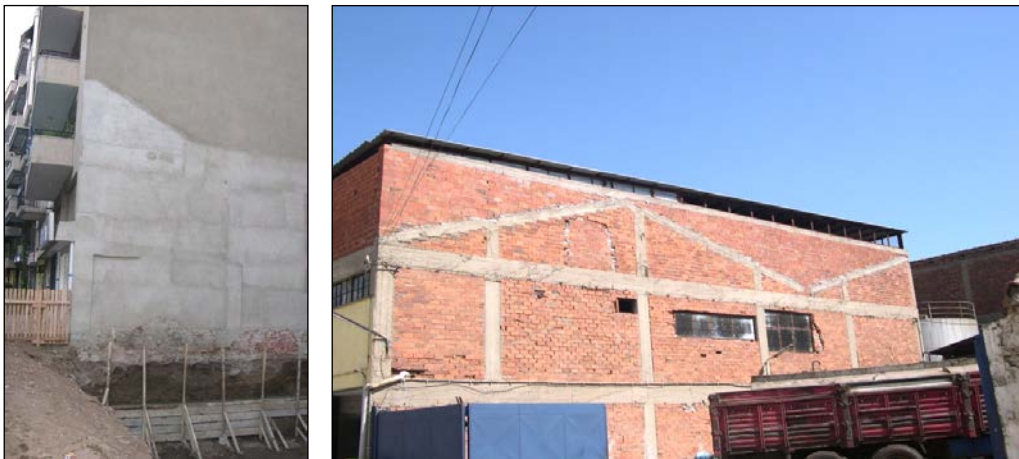
Figure 3. A 5-storey building without a foundation in Şemikler, İzmir (left), an illegal apartment built with the removal of the roof in Çınarlı (right) (Photos; Anonymous, 2009)
