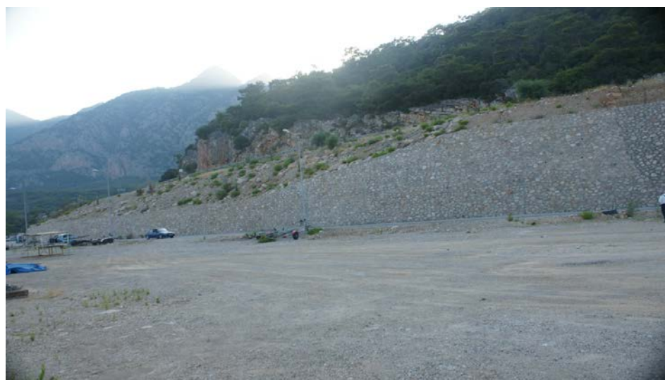
Figure 2. Left Side of Gravity Wall
