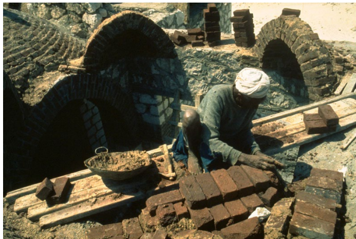
Figure 4. Using mud brick construction techniques, a mason builds an inclined barrel vault (AKTC)
