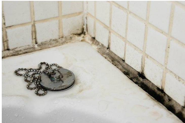
Figure 1. Mold growth on grouted surface in tiled tub surround
